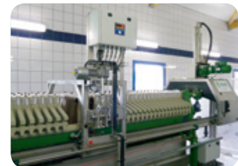
Automatic cake discharge boom
